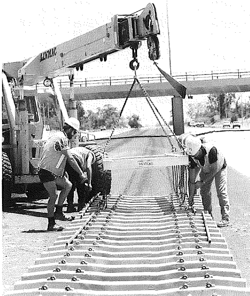
Westrail workers laying sleepers for the new Northern Suburbs Railway. Photograph: Westrail.
